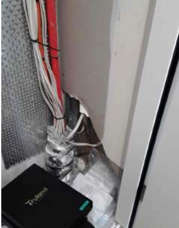
C 190 – Upper ground level, service riser
