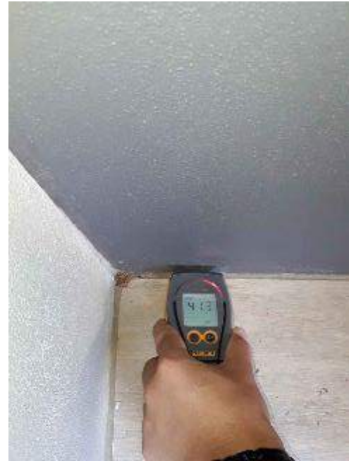
U 306.17 – Unit 306 main bedroom balcony, base of Hebel cladding Elevated moisture to the base of the wall.
