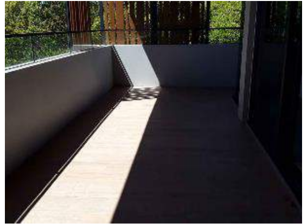
U 304.16 – Unit 30 main balcony, overflow
