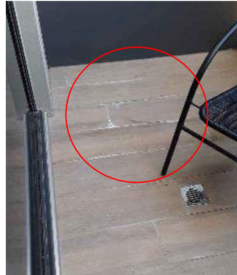
C 306.12 – Unit 306 main bedroom balcony, floor tiles
