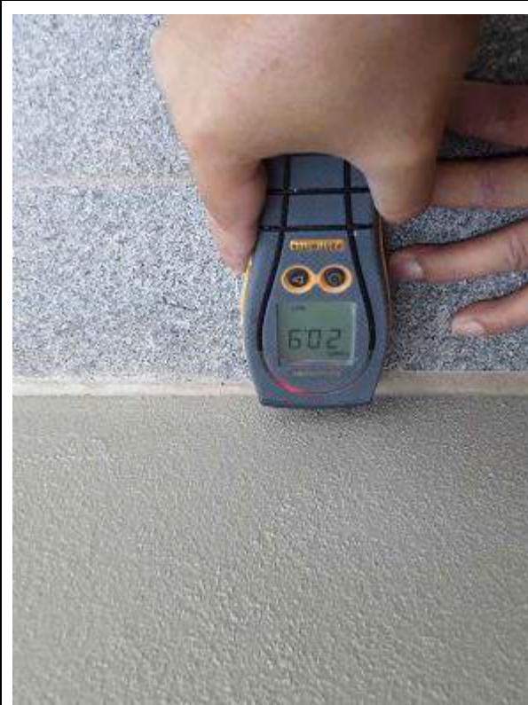
C 4 – Ground floor north entry, Hebel cladding Elevated moisture to base of Hebel wall.
