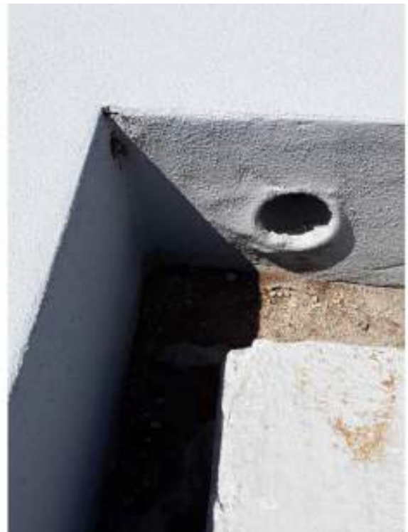
C 161 – Building U, roof overflow
