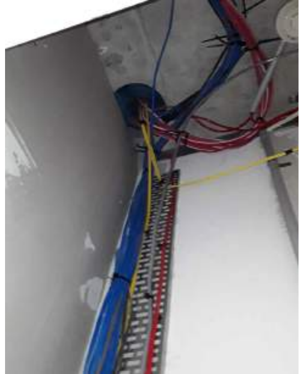
C 192 – Upper ground level, service riser
