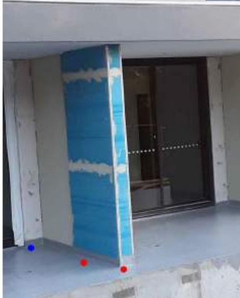
C 10 – East facade, balcony cladding Hebel with no cavity drains (blue).
