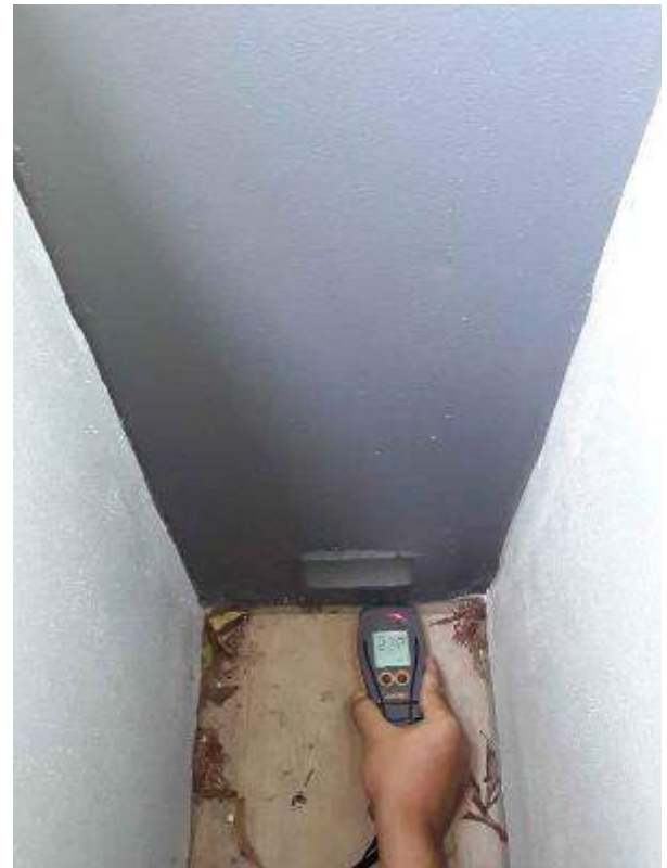
U 304.12– Unit 304 bedroom 2, FC cladding Cladding does not have a drainage provision.
