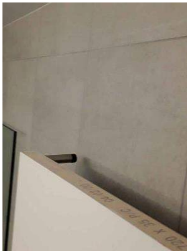
U 304.6 – Unit 304, bathroom top of the door
