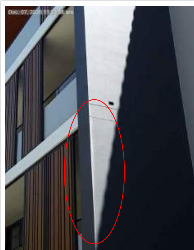
C 50– South facade (Mitchell Avenue), cladding Efflorescence.
