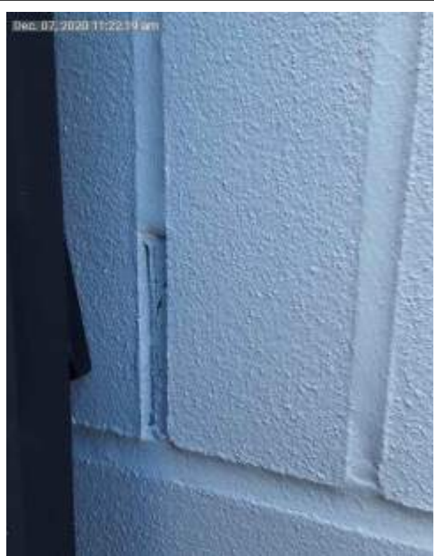
C 25 – East facade, Hebel cladding Drainage provisions are partly covered throughout the facade.
