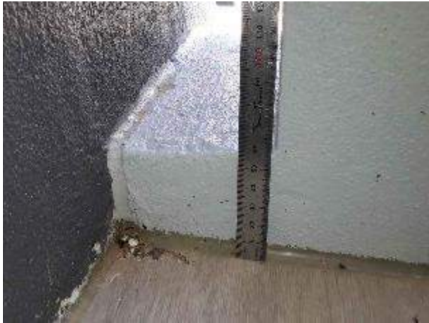
U 306.20 – Unit 306 main bed balcony, overflow
