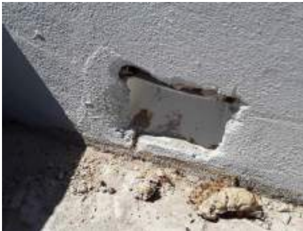
C 156 – Building L, roof overflow
