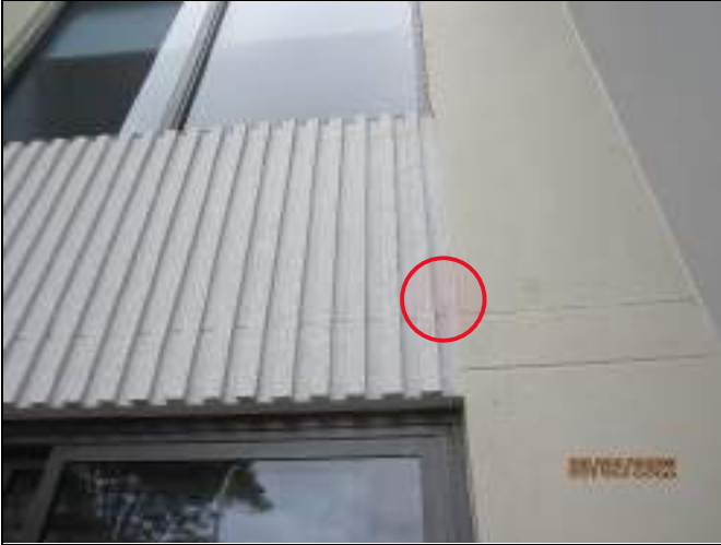
Weep hole drainage painted over above sliding door to bedroom2 Unit G05
