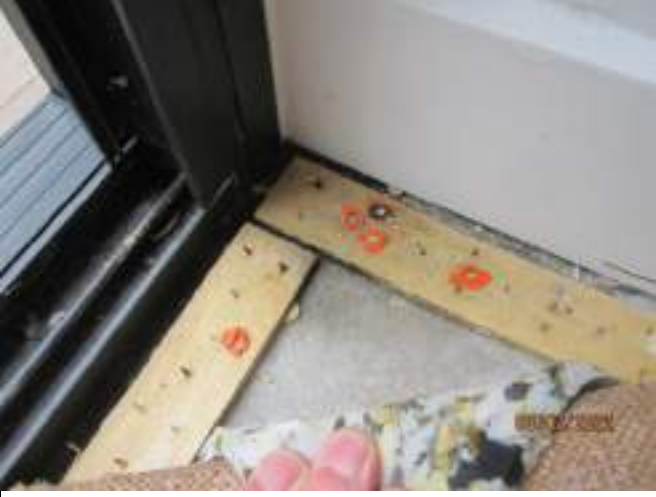
Moisture from rain penetrating interior to western side of sliding door bedroom 2
