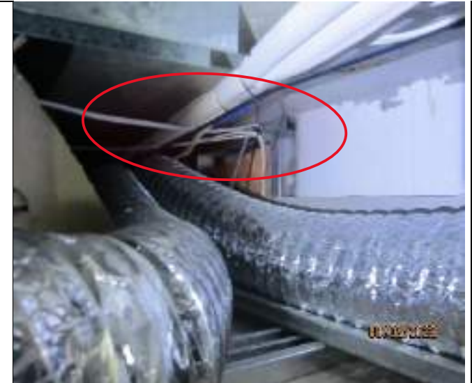
Images showing missing fire separation to common wall to west of location from ceiling access
