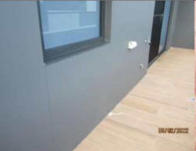
Location of moisture seepage and efflorescence staining to western side of southeast sliding door
