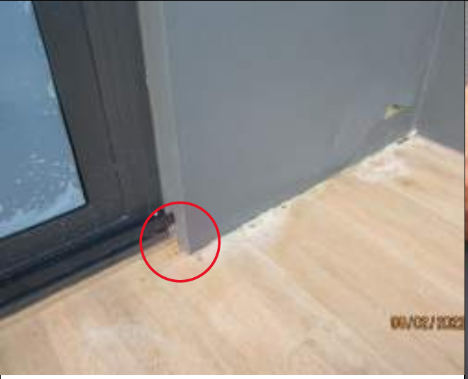
Location of water penetration
