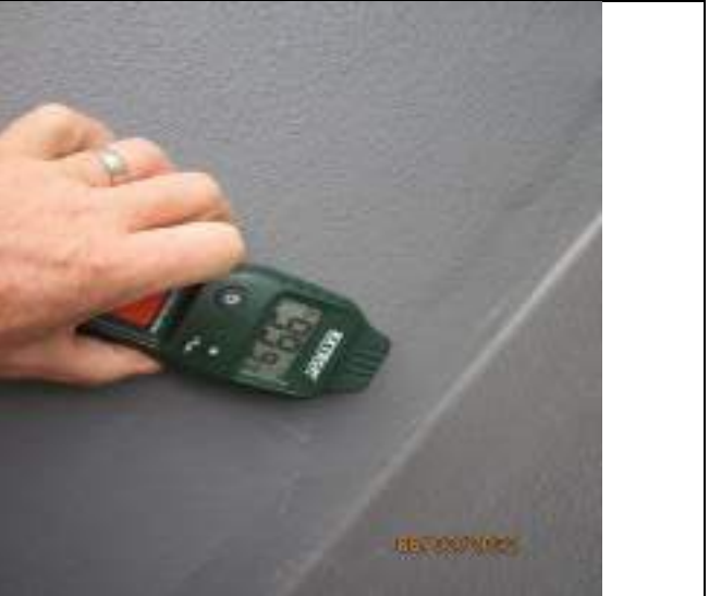
Highly elevated level of moisture indicated to surface of rendered Hebel wall at southeast corner
