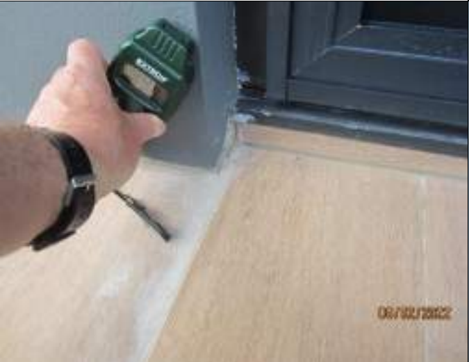
Evidence of moisture seeping and efflorescence staining at western side of southeast sliding door
