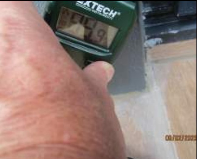
High level of moisture indicated to Hebel rendered wall above location of water seepage and efflorescence staining
