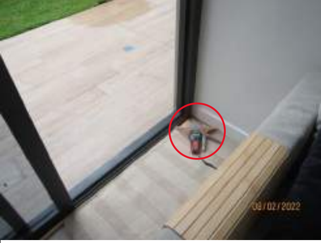
Location of rainwater penetration to western side of sliding door bedroom 2
