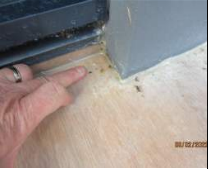
Water seeping at junction of wall and sliding door to southeast following rain
