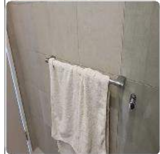
Ensuite shower screen door is striking metal towel rail
