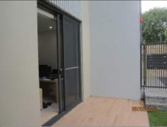
Location of bedroom 2 sliding door Unit G05 looking east and light weight wall adjoining main entry ramp
