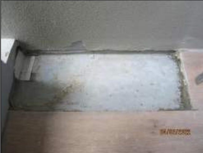
Tile removed adjacent to northeast column and overflow to balcony
