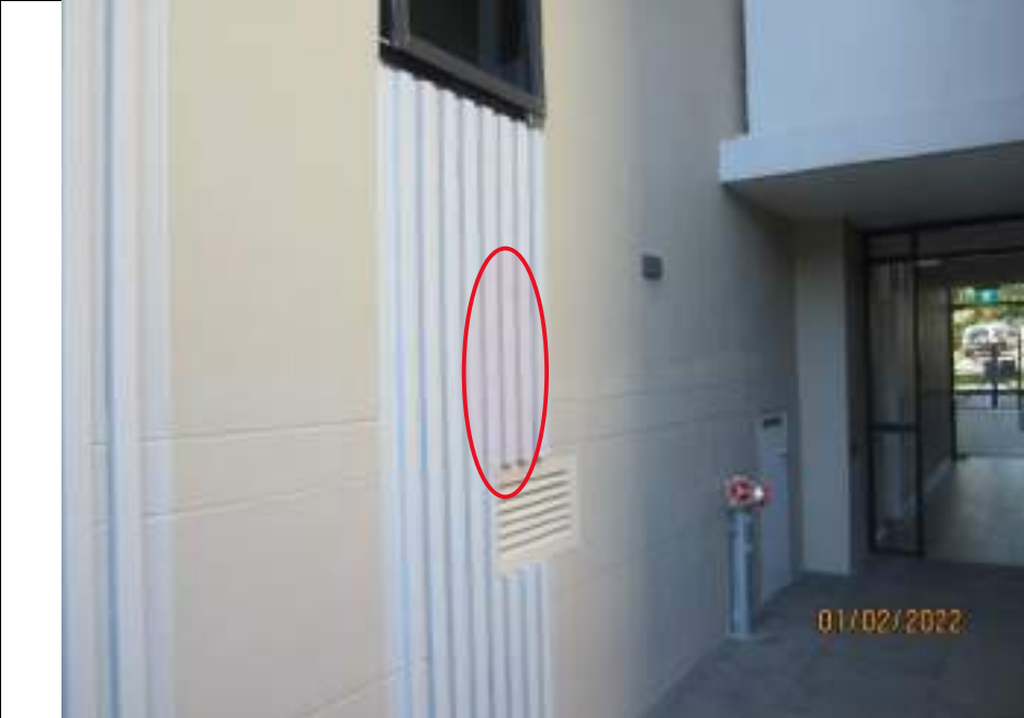
Location of defects western façade Building L northwestern side of entry
