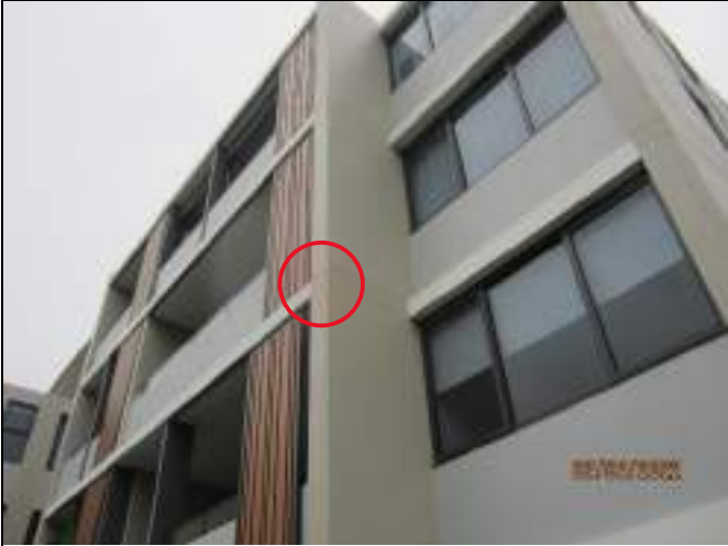
Evidence of rainwater leaks above northwest lightweight balcony wall to Building U
