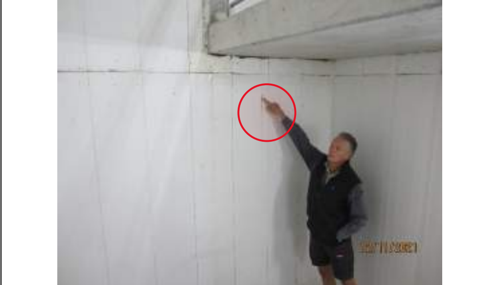
Location of water penetration at eastern wall on stair landind above basement level 1
