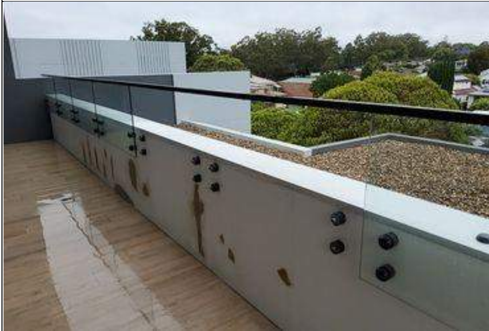
Image showing balustrade metal capping and evidence of Builders repair to unit 403 to southern side of balcony terrace
