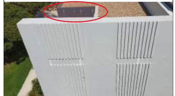
Evidence of efflorescence staining to parapet wall at roof level
