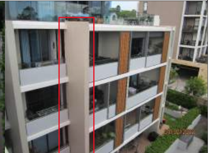
Location of cantilevered concrete deflection, distortion of building elements and water leaks to north east of Building U
