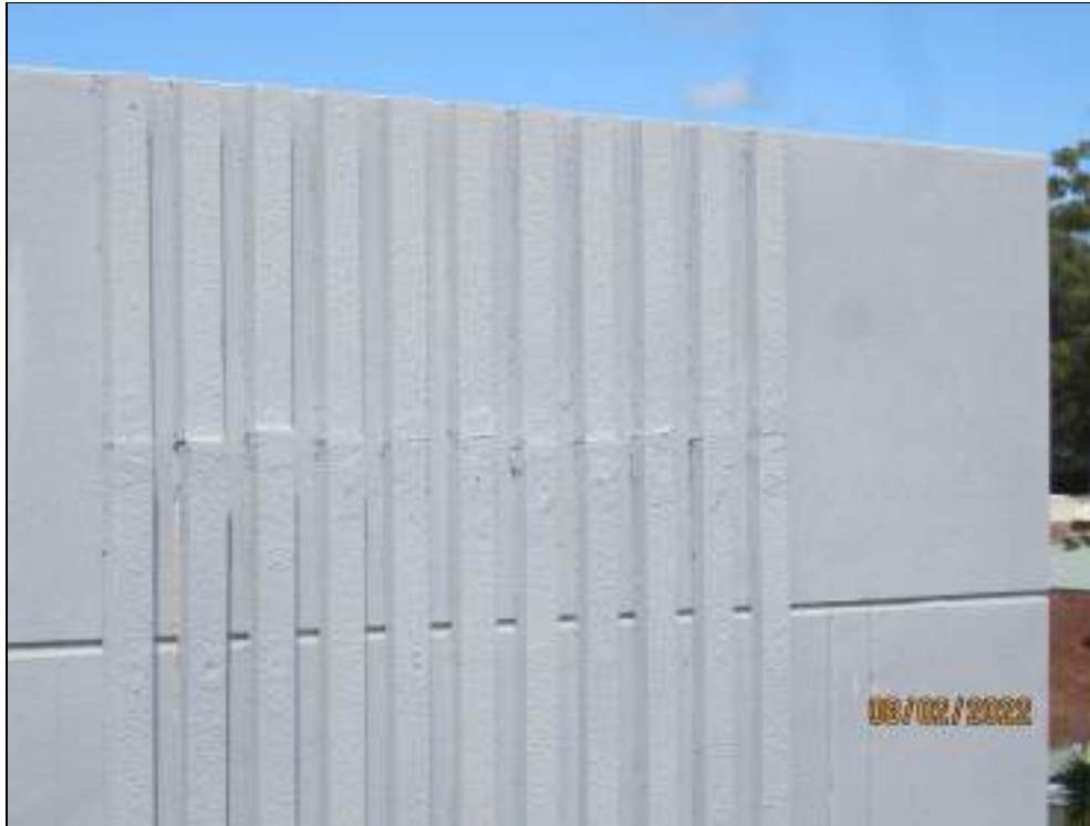
Evidence of poor workmanship to install to Building L façade battens above southern entry
