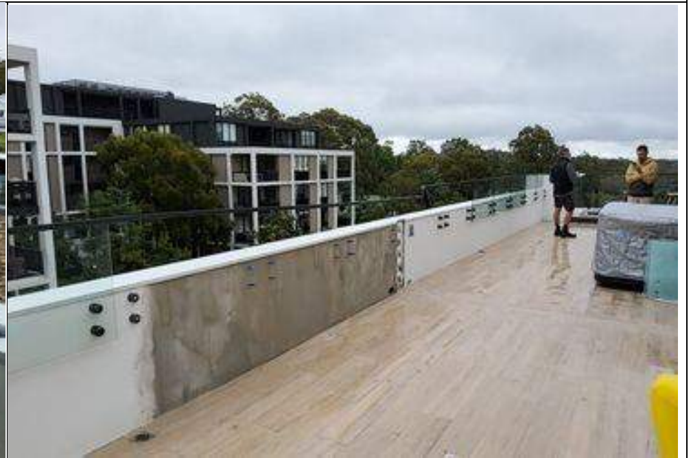
Image showing balustrade metal capping and evidence of builders repair to unit 403 to western side of balcony terrace
