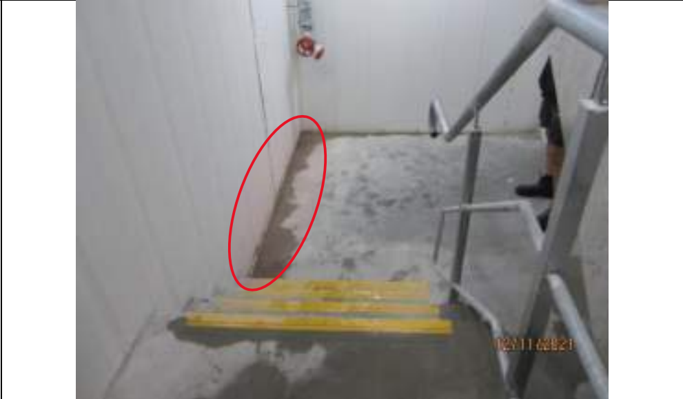
Water penetrating base of Dintel to southern wall in Stairway 2 at Basement 2 level
