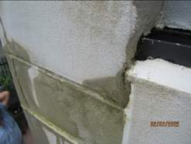
Evidence of water flood test penetrating column to northeast column of unit 107
