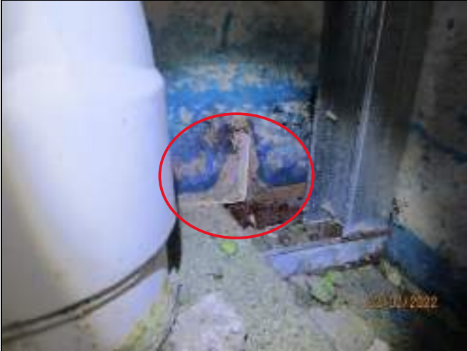
Evidence of water flood test penetrating interior of column to northeast column of unit 107. PVC angle used to form vertical termination penetrating lining to column.
