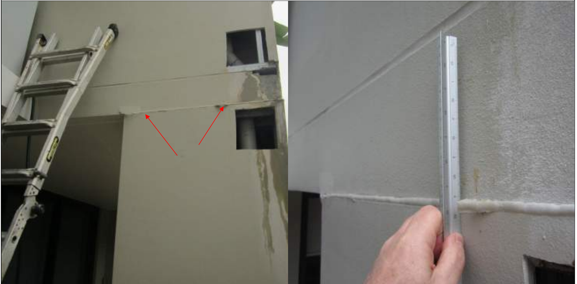
EVIDENCE OF DEFLEXION (SAG) TO CANTILEVERED CONCRETE SLAB CAUSING DISLODGE- MENT OF SEALANT AND DAMAGE TO RENDERED LININGS TO NO STRUCTURAL LIGHT WEIGHT WALL AT GROUND LEVEL TO NORTHEAST COLUMN OF BUILDING U.
