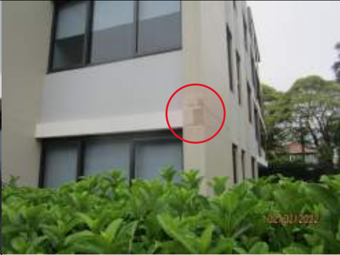
Evidence of rainwater leaks to northwest corner of Building U
