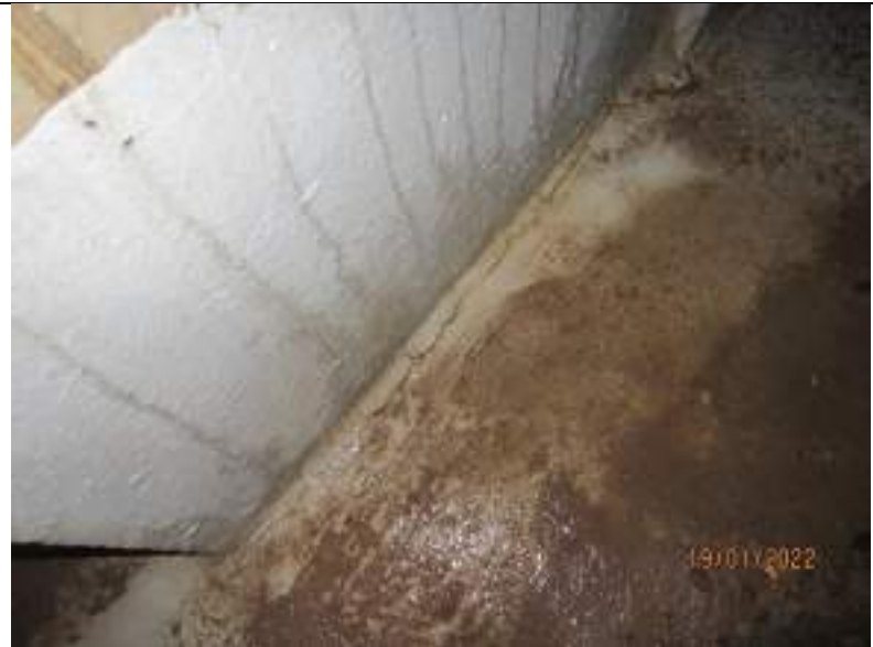
Evidence of bond breaker failure to waterproofing repair at rear of southwest wall of switch room
