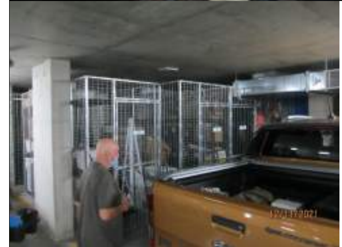
Evidence of mould on surface of materials in storage to southwest corner of Basement 2
