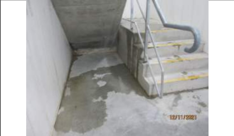
Water pooling on floor at Basement 2 level in Stairway 2 orinating from water leak to northern wall above stair landing
