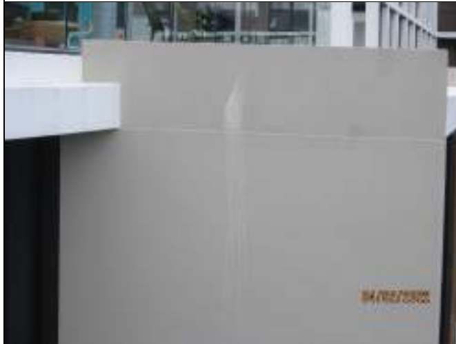
Evidence of water penetration to linings on northeast column to Building U
