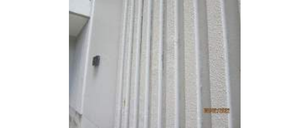
Evidence of cracks and gaps to battens fixed to southeastern side of entry
