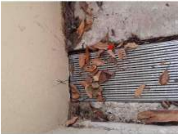
Gaps to drain at base of Fire stair door
