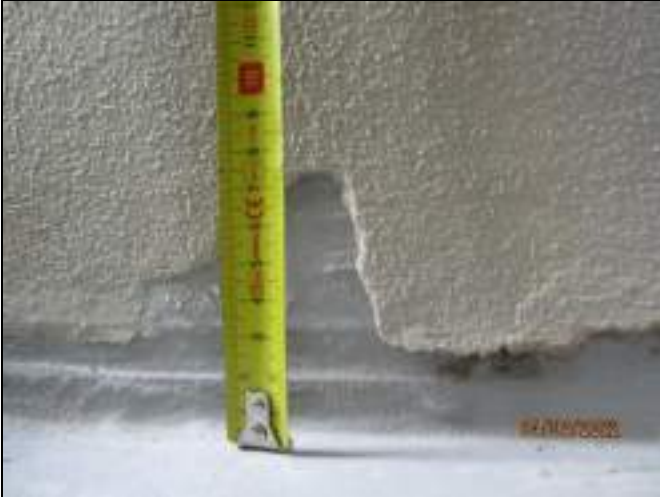
Height of upturn to waterproofing to northeast column above 70mm
