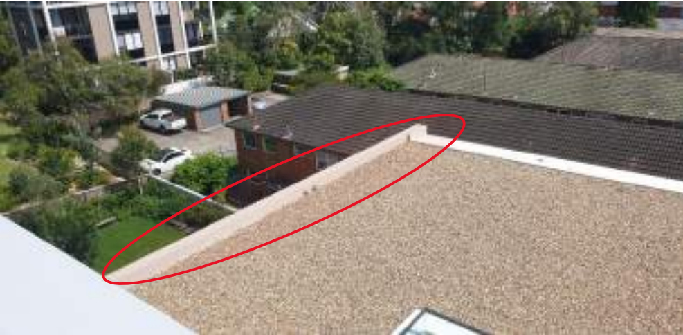
No flashing or waterproofing provided to building parapets
