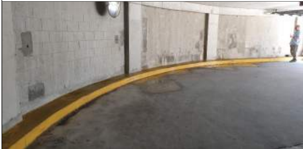
Image of northern retaining at basement entry with evidence of waterproofing repair
