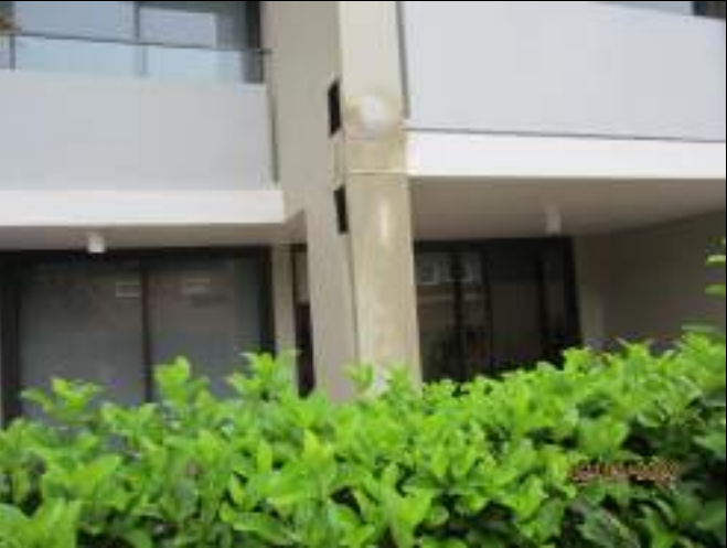
Evidence of water flood test penetrating column to northeast column of unit 107
