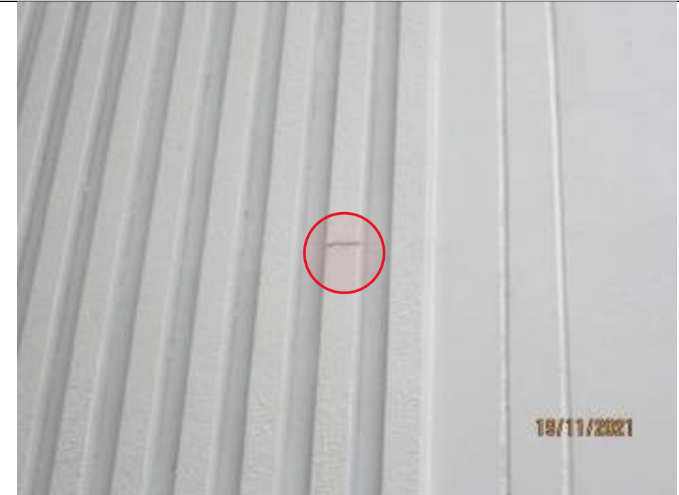
Evidence of damage to aerated concrete battening to eastern wall of main entry
