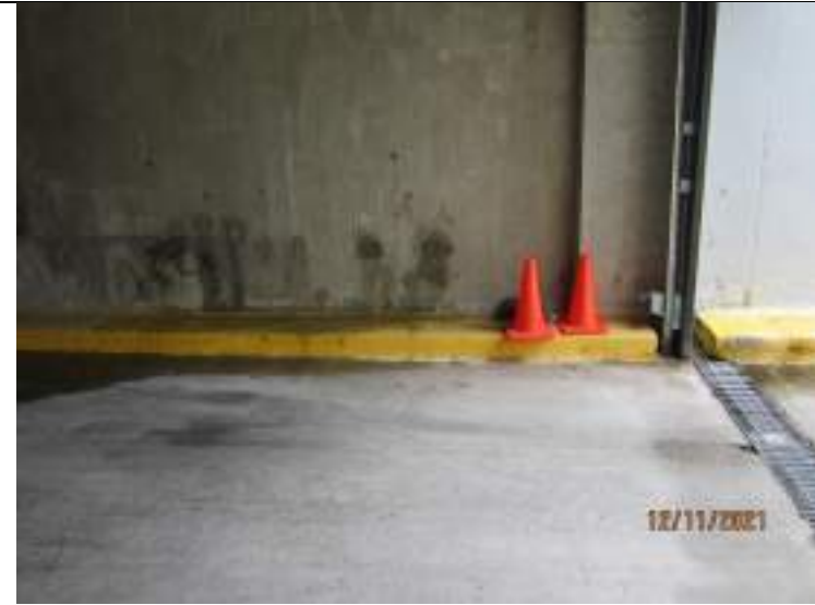
Evidence of failed waterproofing repair to water leaks
