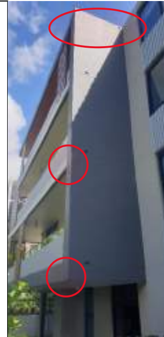
Location of moisture penetration and efflorescence staining
