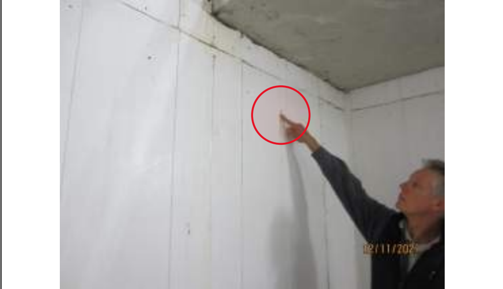
Water penetration identified at stair landing on eastern wall above basement level 1
