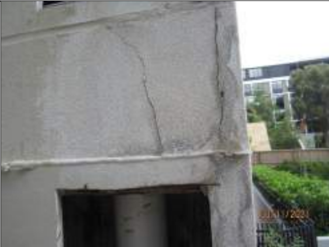
Evidence of moisture damage to northeast corner of column
