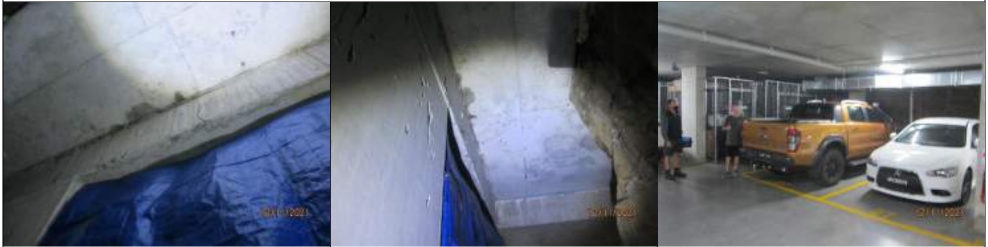
Tarp installed by lot owner to prevent moisture damage originating from slab to southwest storage of Basement 2
