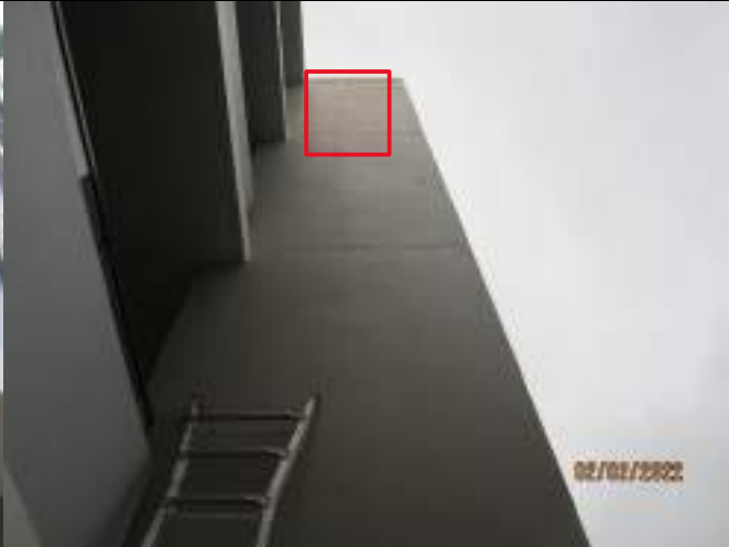
Evidence of rainwater leaks above northeast lightweight wall to Building U
