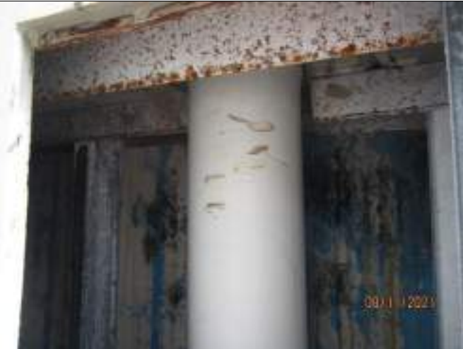
Evidence of corrosion to steel frame to interior of column exposed on northeast corner.
