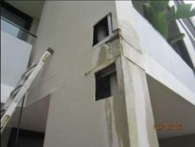
Evidence of water flood test penetrating column to northeast column to balcony of unit 107
