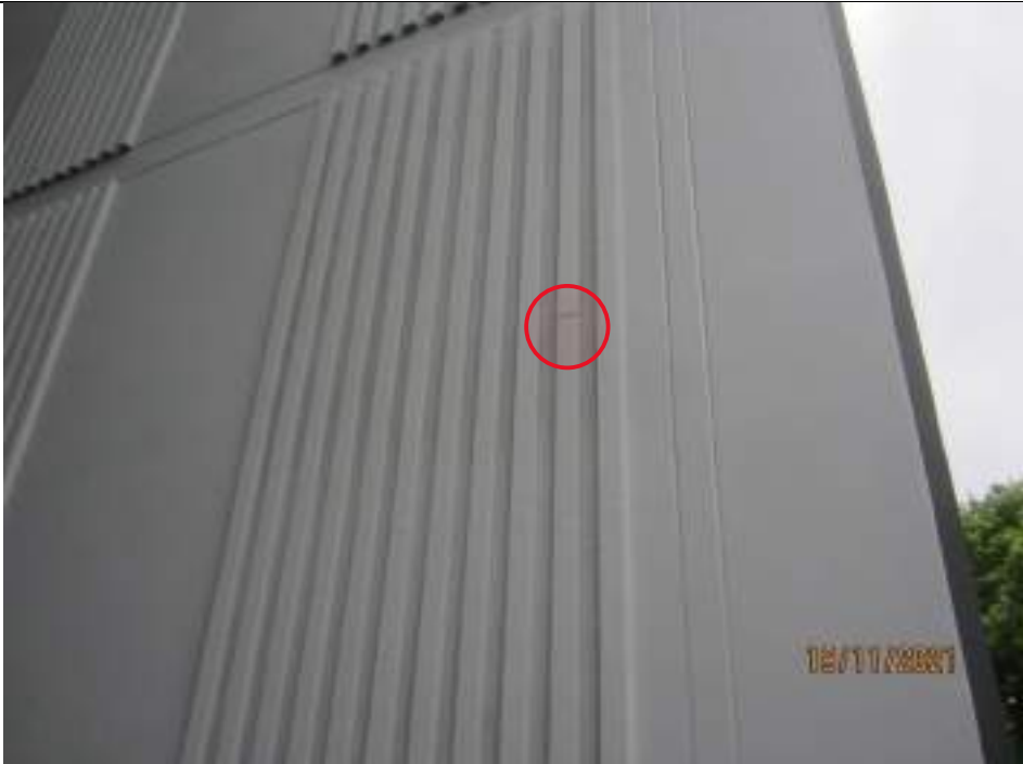
Evidence of damage to aerated concrete battening to eastern wall of main entry
