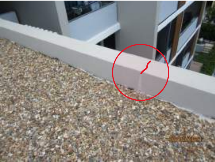
Efflorescence staining to western side of building L façade above entry inline with crack on top of façade parapet indicated in red
