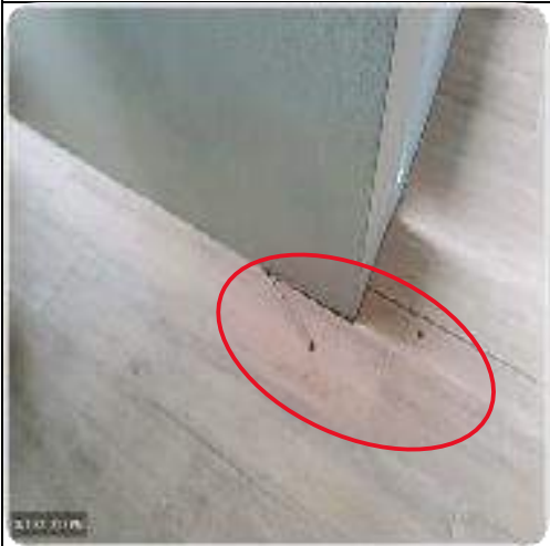
Image showing flexibale sealant that removed by the Builder to conduct dye test at the junction on the southwestern corner of the column to unit 107 that was reported at the time inspection to the Author by the owner occupant of unit 107.
