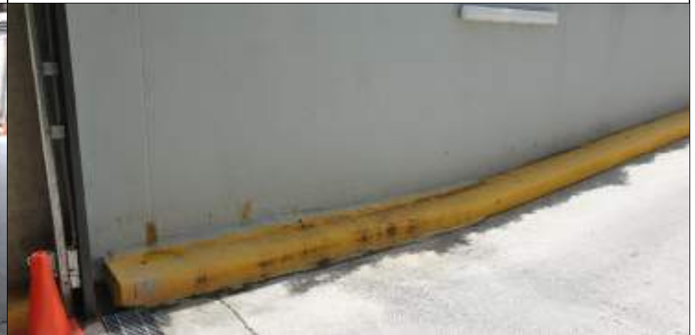
Evidence of waterleak to base of retaining wall on northern side of basement entry
