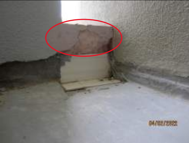
Overflow built up above PVC has not been waterproofed
