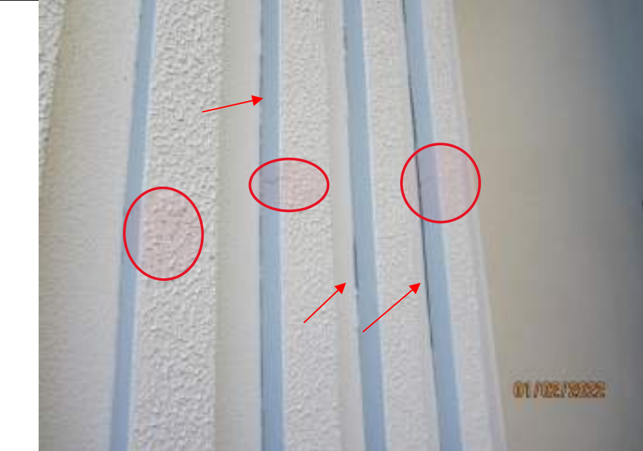
Image showing cracks and gaps to battens
