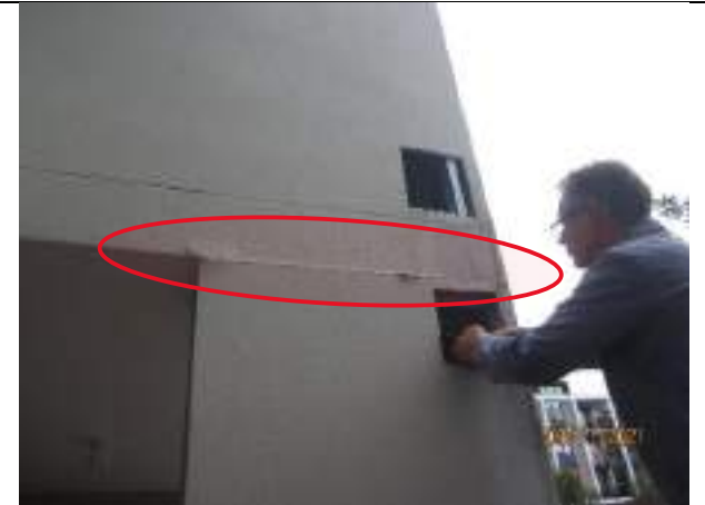
Images showing openings cut in column to northeast corner reported by occupants to have been done by the Builder., and evidence of damage caused due to deflexion of cantilevered concrete slab.
