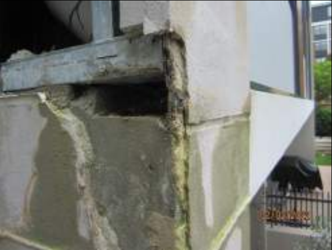
Evidence of water flood test penetrating column to northeast column of unit 107
