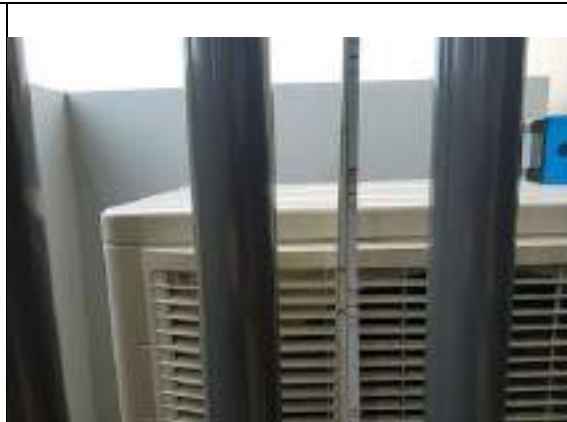
Unit 302 Air conditioner height approximately 550mm
