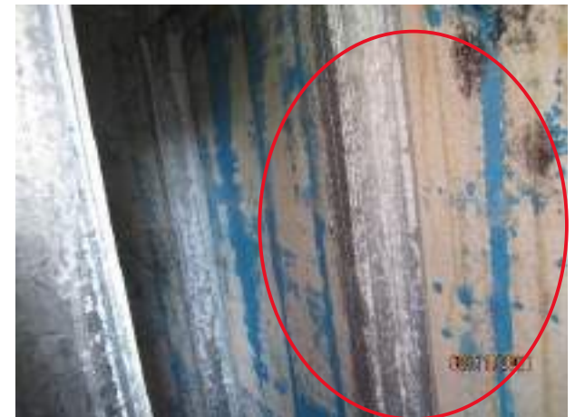
Yellow staining to interior surface of cladding
