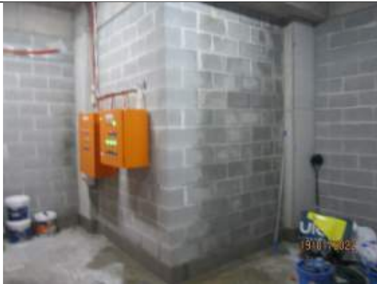
Image showing moisture penetrating southwestern masonry wall above waterproofing membrane
