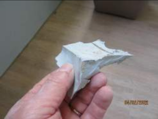
No bond breaker or fillet provided at horizontal junction
