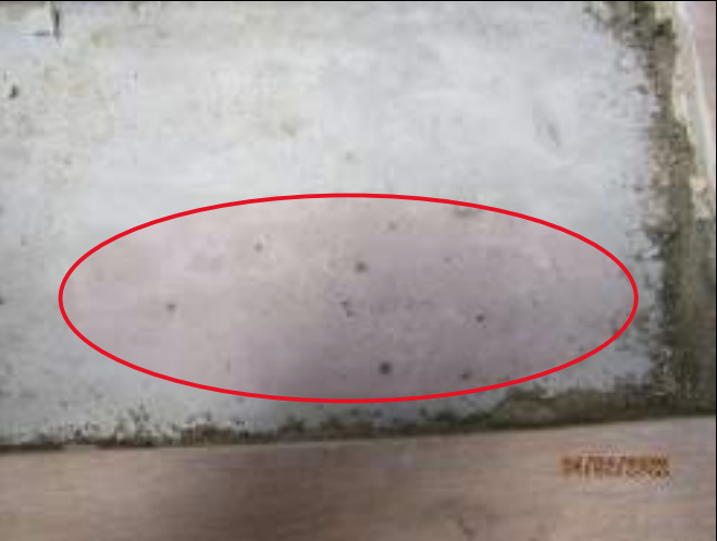
Evidence of pin holes to waterproof membrane
