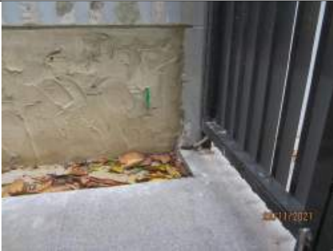
Weepa's installed to base of wall have no useful function
