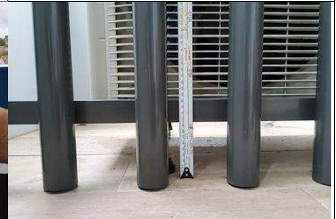
Unit 302 height of horizontal rail on barrier approximately 140mm
