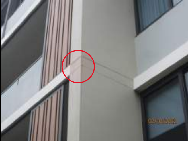
Evidence of rainwater leaks above northwest light weight balcony wall to Building U
