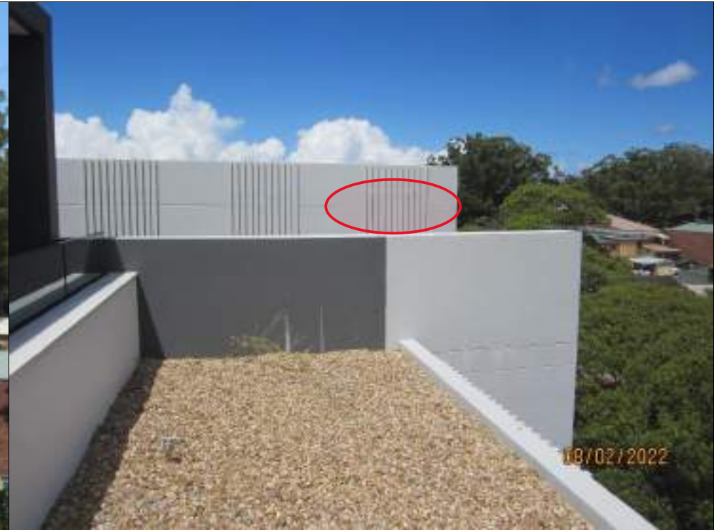
Location of poor workmanship to Building L above main entry
