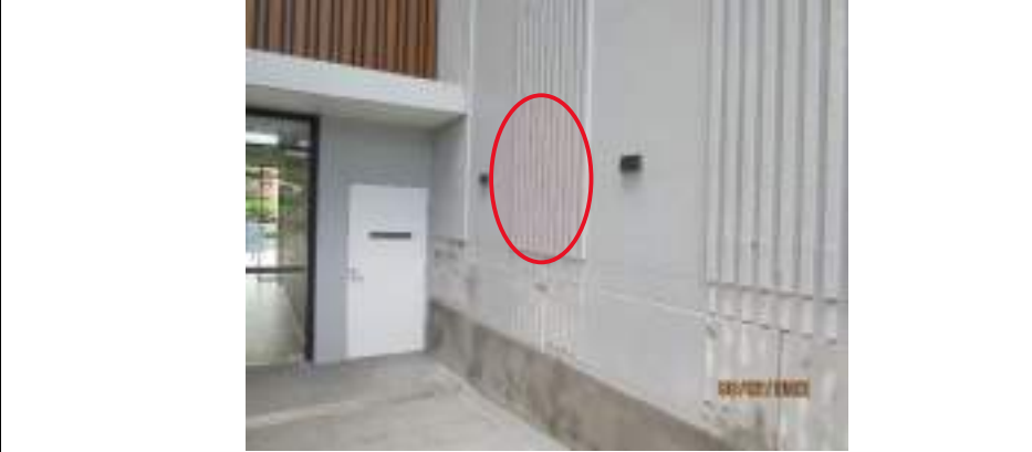
Location of defects western façade Building L southeastern side of entry
