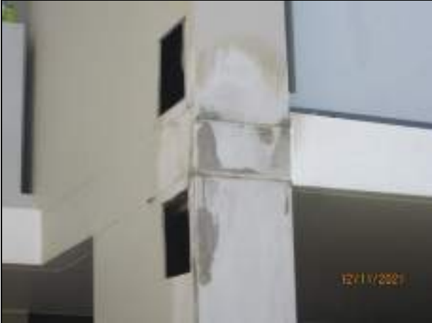
Evidence of moisture penetration following rain on day of inspection
