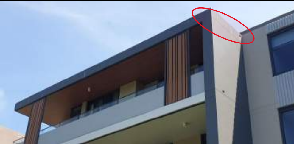
Location of efflorescence staining to building façade above balcony to unit 305
