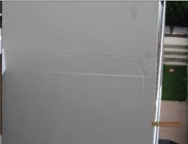
Evidence of water penetration and deflexion in cantilevered concrete slab northeast balconies of Building U
