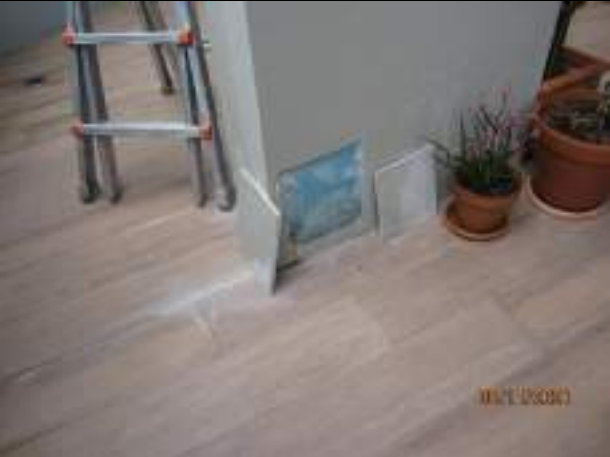
Column material exposed to northwest side of the column reported to the Author at the time inspection to have been done by the Builder.
