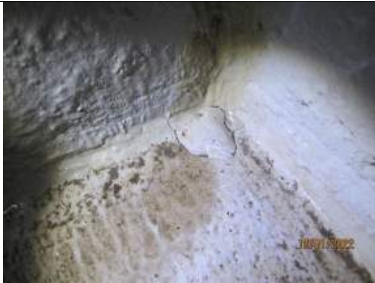
Evidence of bond breaker failure to waterproofing repair at rear of southwest wall of switch room
