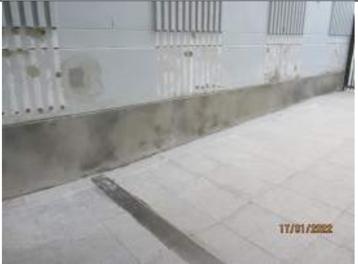
Render finish applied to waterproofing is drummy
