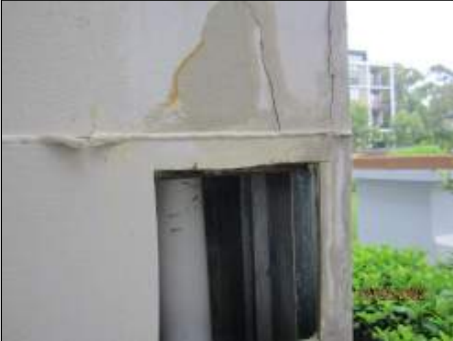
Evidence of water flood test penetrating column to northeast column of unit 107
