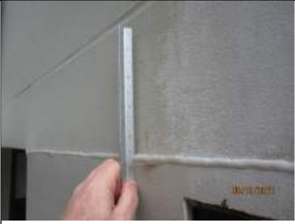
Evidence of rupturing of gasket sealant to horizontal joint and distortion to alignment of building elements caused due to deflexion of cantilevered concrete slab
